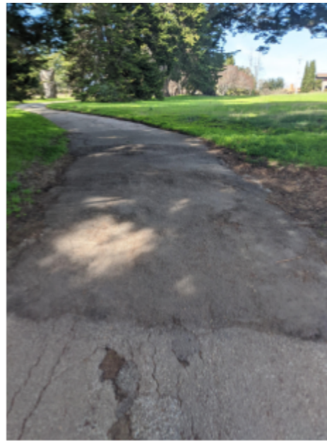
Figure 3.2.2: Image of poor asphalt conditions along Cardiff Path
