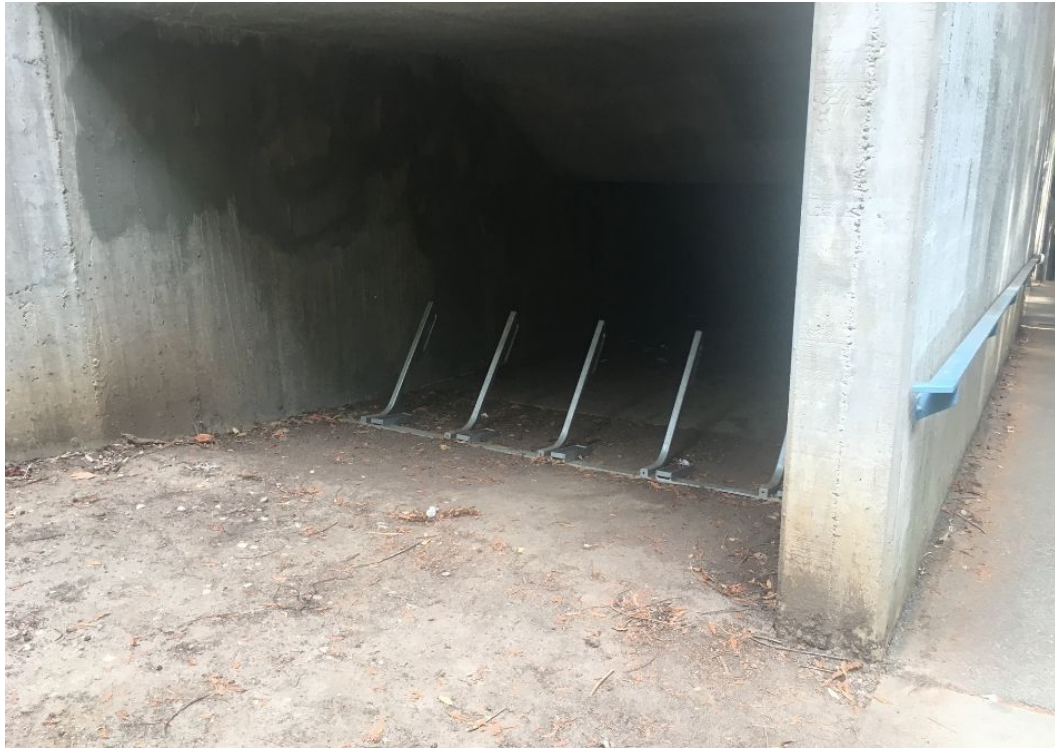
Figure 8: Example of Poor Location (Classroom Units)
